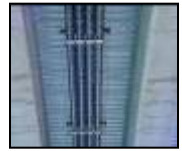
UNDER BRIDGE CONDUIT SYSTEMS
