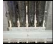
BRIDGE ATTACHMENT HANGERS & SUPPORTS
