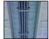
UNDER BRIDGE CONDUIT SYSTEMS
