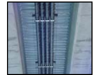
UNDER BRIDGE CONDUIT SYSTEMS
