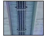
UNDER BRIDGE CONDUIT SYSTEMS
