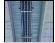
UNDER BRIDGE CONDUIT SYSTEMS
