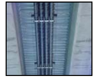
UNDER BRIDGE CONDUIT SYSTEMS
