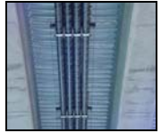
UNDER BRIDGE CONDUIT SYSTEMS
