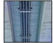
UNDER BRIDGE CONDUIT SYSTEMS
